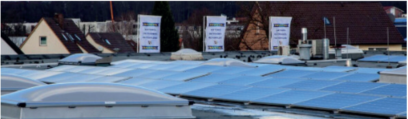
PV system at the Werther plant: Efficient power generation since 2016 and an active contribution to climate protection
